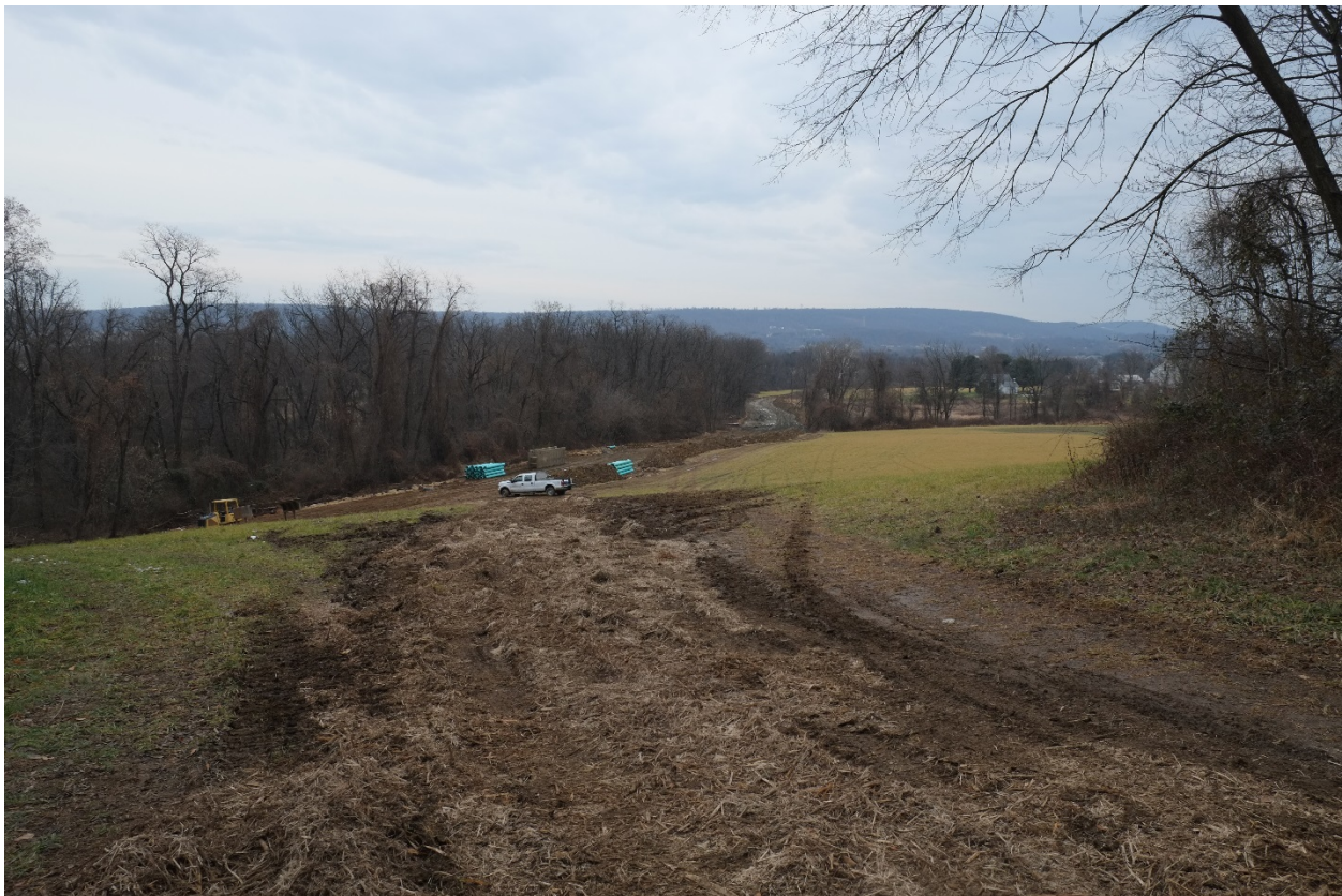
Figure 9. Photograph taken on 12/11/2017 from the SW corner of the Wiest block showing the footprint of work on the sanitary sewer. View is to the north. Shultz farmhouse is visible in the background to the east of the constructed equipment/pipeline access road.
